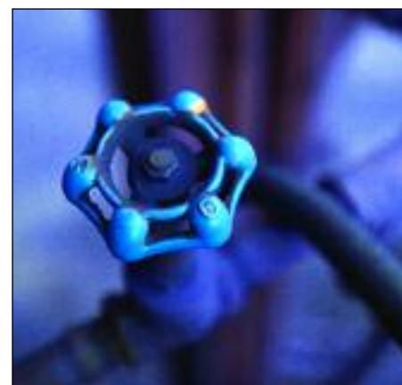
Sometimes installing one inexpensive new valve can save thousands of dollars.
